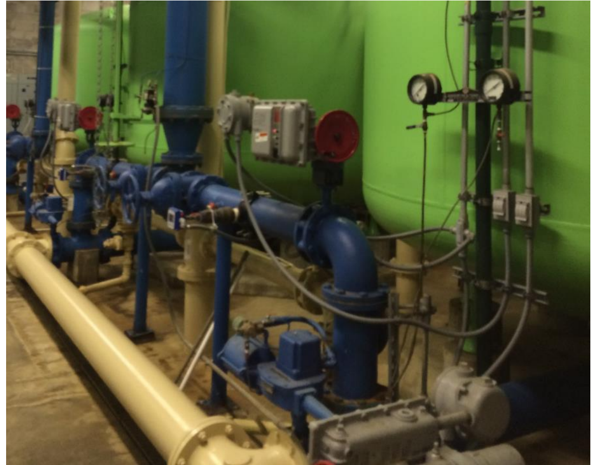
Existing filter piping, valves and actuators
